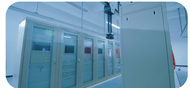
Protection room track robot
