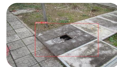
Damaged or missing cover plate
