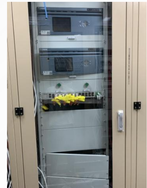
Figure 6 Front wiring cabinet
